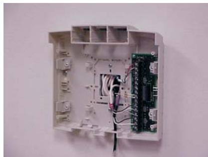
Figure 14: Installed termination module
