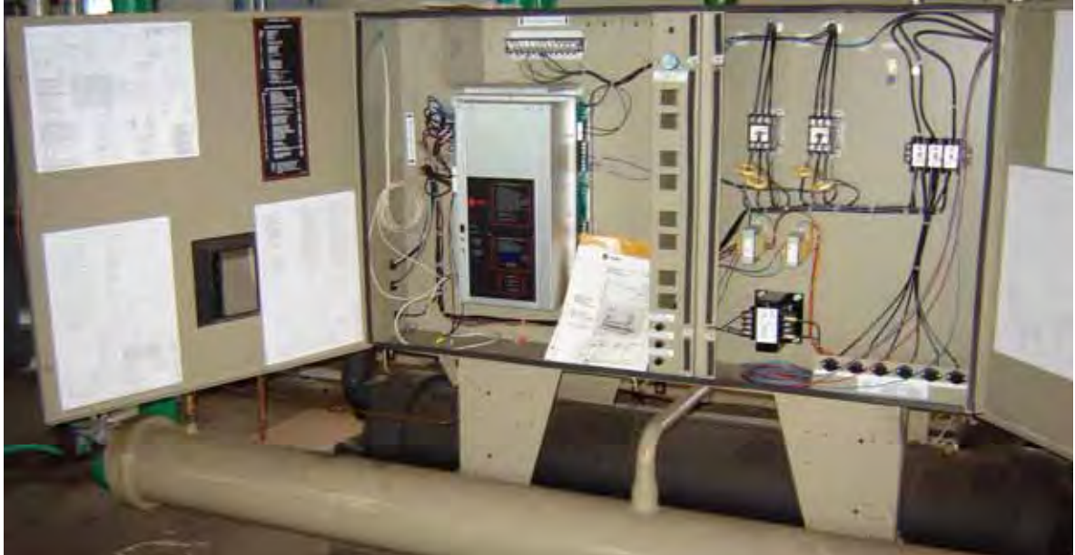
Figure 1. Typical water cooled panel before removal
