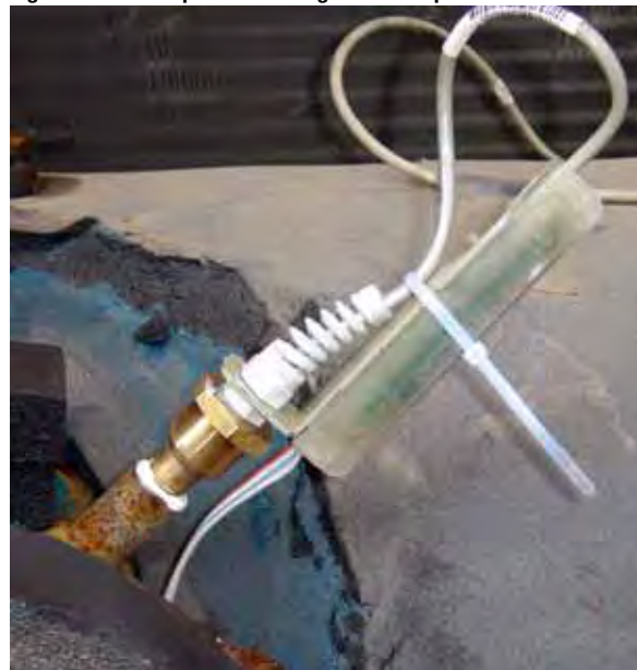
Figure 5. New evaporator leaving water temperature sensor
