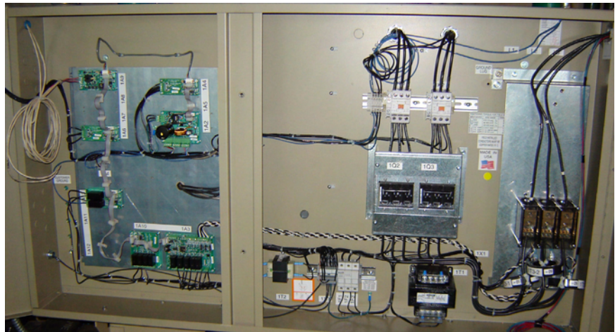
Figure 3. Water cooled 30 ton control panel with CH530 components
