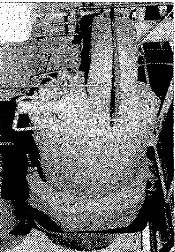
Chiller with HUSH COVER™ Blankets
