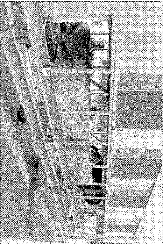
Chiller with HUSH COVER™ Blankets
