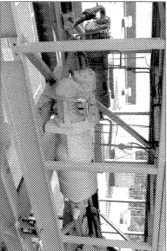
Untreated Chiller Compressors
