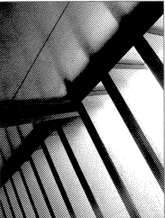
Overhead exhaust parallel baffles shown from inside looking up
