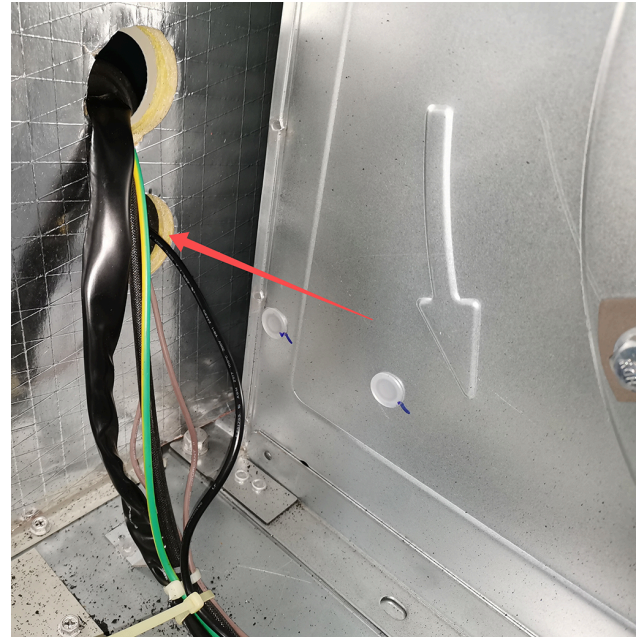
Figure 8. Supply fan blower section
