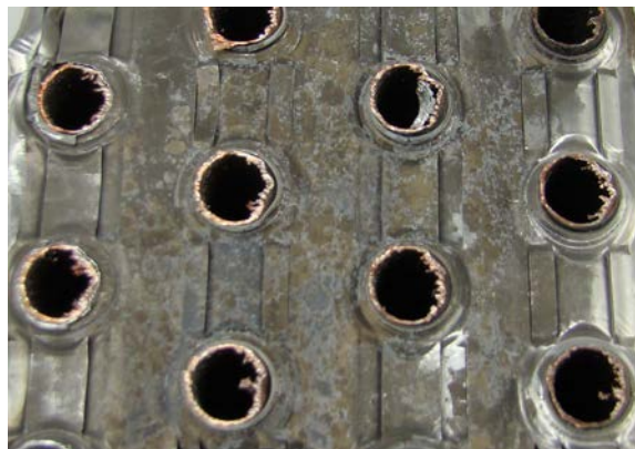
Figure 3. A close-up view of the fin surface shows the blackening and corrosion phenomena.
